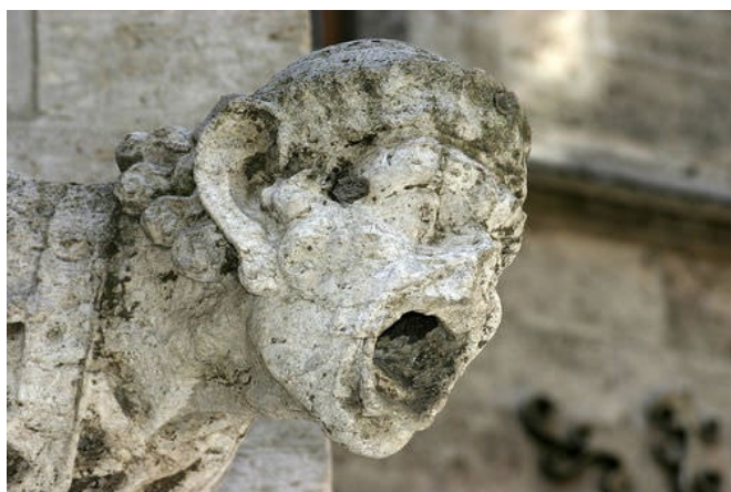
Figure 11.3 A gargoyle that has been damaged by acid rain (credit: chem.libretexts.org).
